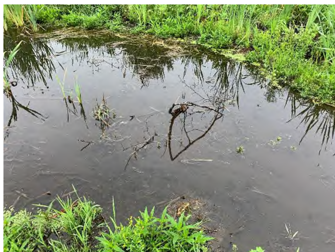
Knight's Brook – 3 (Above Duct Bank in Brook)
